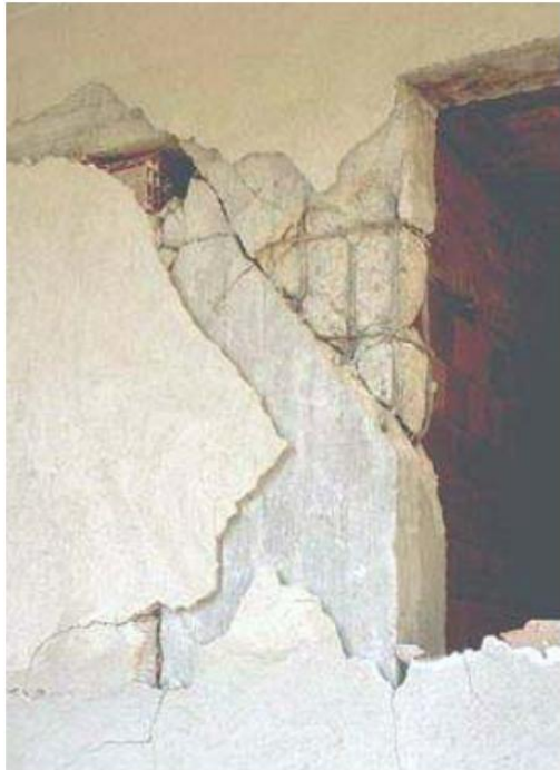
Shear failure in KOCIZN, KOCYPT
