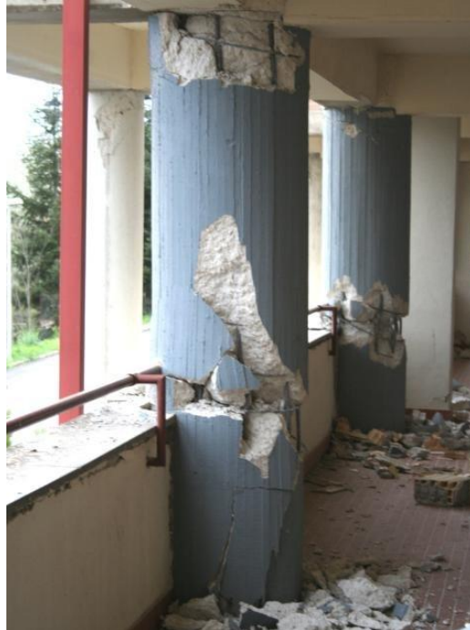
Typical shear failure of circular column
